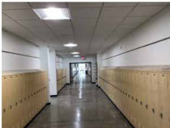
Installed All ACT
