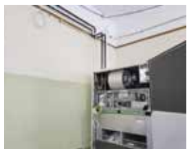
3rd Floor Classroom Unit Ventilator
