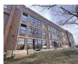
New Window System
